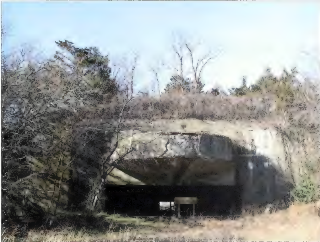
Figure 3.49. View looking west at emplacement #2, Battery Mills. Above the emplacement, large spalling areas on the concrete canopy result from infiltration of water and seasonal freezing and thawing (Olmsted Center, January 2009).
